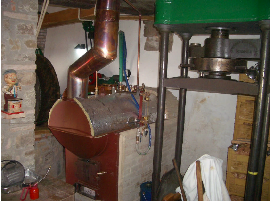
A boiler set up in a working situation
